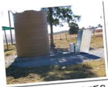
BUILDING WATER STORAGE TANKS
